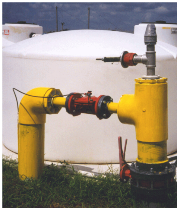
Figure 13. Hydraulically actuated control valve with vacuum and pressure relief valves downstream.
