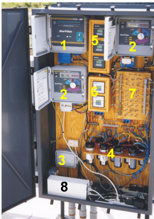
Figure 14. In-field controls for a centrally-controlled citrus irrigation system including: 1) on-site communication, data storage, and control device; 2) valve, pump, and accessory controllers; 3) phone connection; 4) sensor decoders; 5) flow monitors; 6) pressure and water level monitors; 7) manual over-rides; 8) power conditioning and surge protection.
